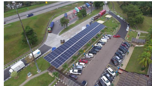
Aerial view of Solar PV system installed at Machap RSA Northbound
